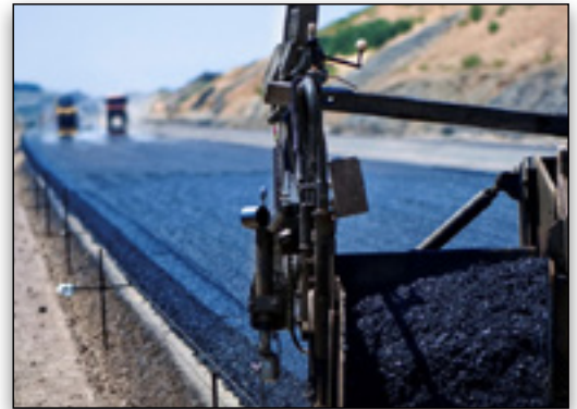
Grontmij used MXRoad and OpenRoads to deliver template-based designs allowing all parties to virtually review full pavement layers and construction depths.
