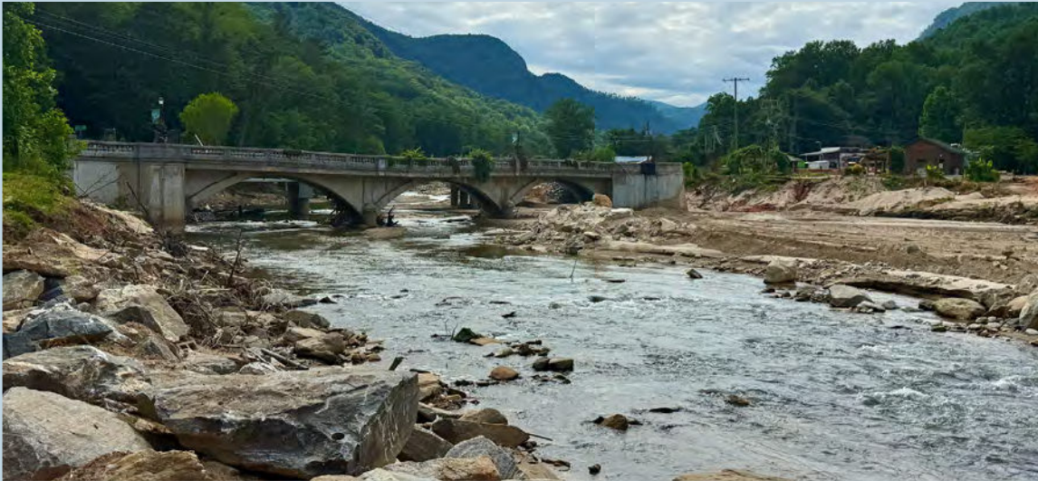
Figure 7. Flooding following Hurricane Helene disrupted infrastructure in Western North Carolina
