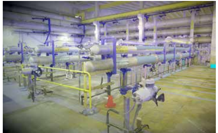
The reality mesh provided a detailed representation of every area and angle of the project, eliminating the need to travel to the worksite. Image courtesy of Jacobs Engineering.
