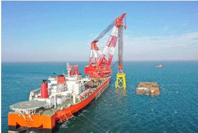
Caption: The deep-sea wind farm project is the first in the global offshore wind industry to adopt the new suction pile jacket foundation.
