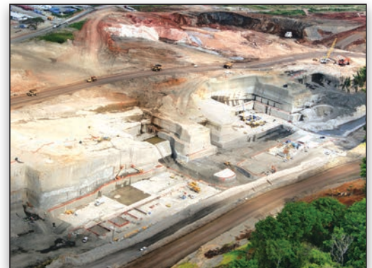
Jan De Nul is engaged in dredging 20 million cubic meters of rock from the Pacific north access channel and the Atlantic entrance.
